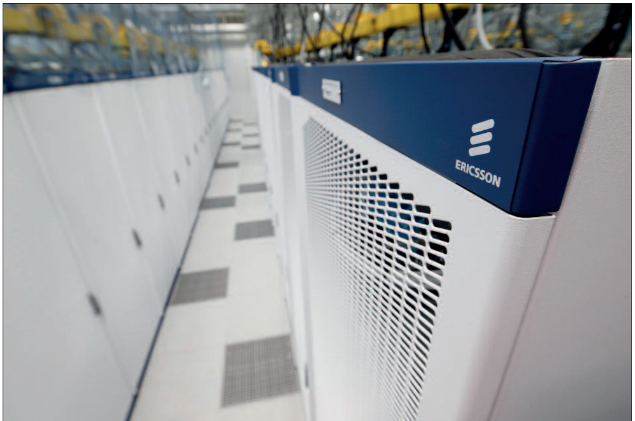
Figure 1: Typical data cabinet utilizing conventional point-of-load power architecture
