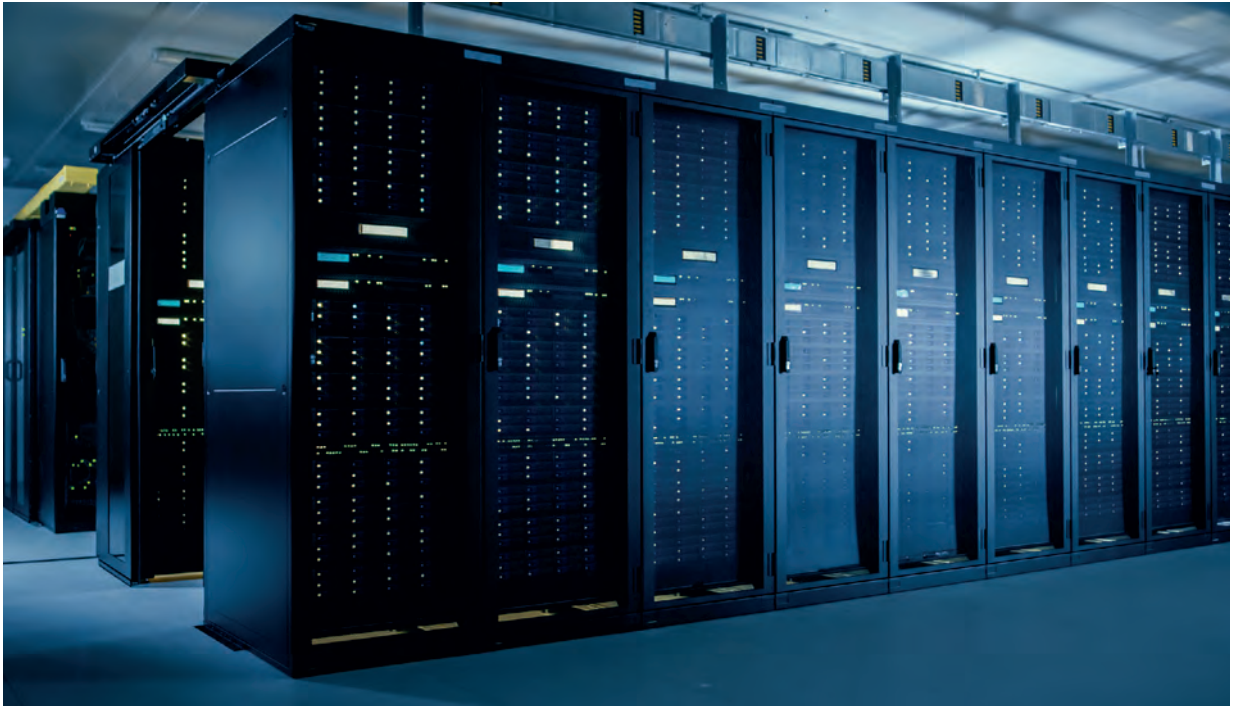
Figure 2: Server racks in a data centre.
