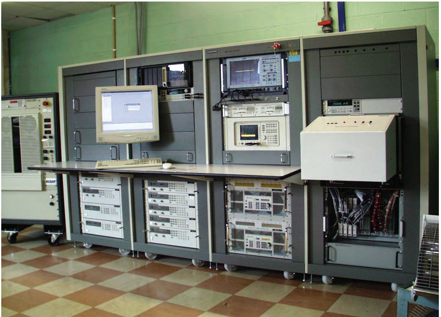
Photo: System ready for refurbishment for online
